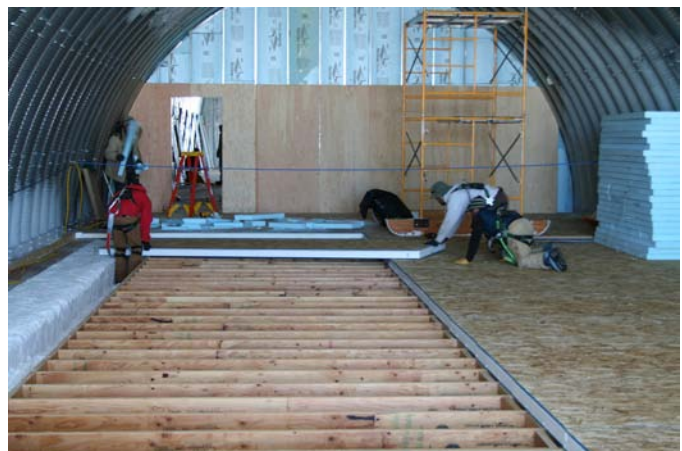
Arch construction crew installing the floor in the core-processing arch. Directly beneath this floor is the core storage trench where all brittle ice will be stored for a year before being shipped to NICL. Photo: J. Souney
